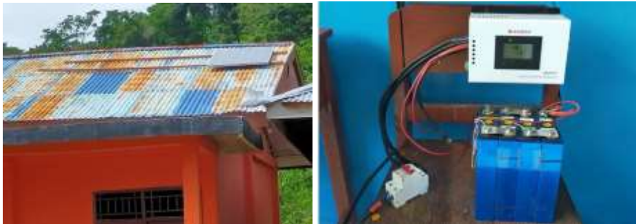
Gambar 14. PLTS 1 (PV 300WP; 2 Aki 100ah, 12V; Inverter 1000W)
