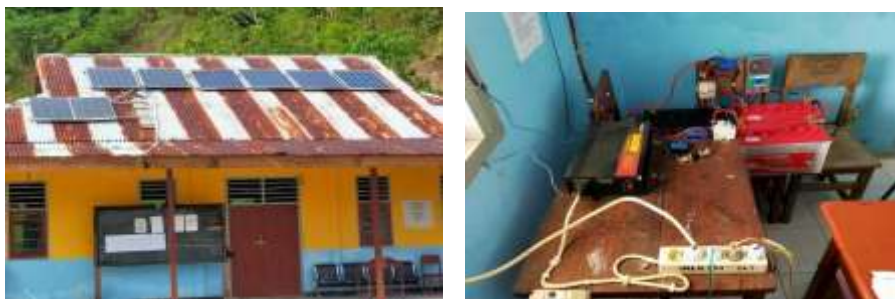
Gambar 16. PLTS 3 (PV 1600WP; 4 Aki 100ah,12V, Inverter 2000W)
