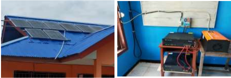
Gambar 17. PLTS 4 (PV 1600WP; 2 Baterai Shoto 100ah,48V, Inverter 3000W)
